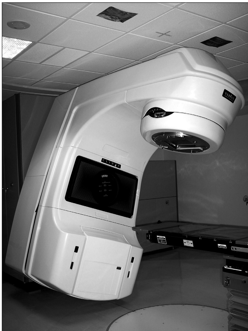
3 External beam therapy equipment (linear accelerator)
